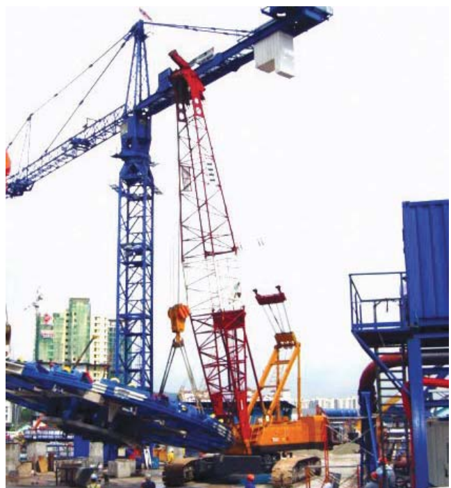
Our 500-ton heavy crane lifting the TBM Cutter head weighing 282 tons for KL SMART project in Malaysia.
