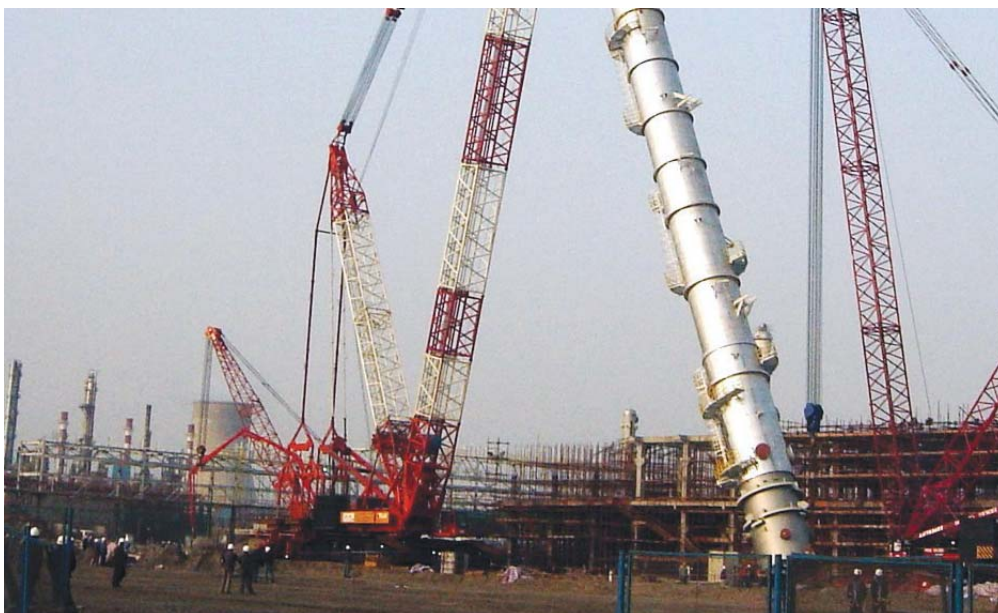
Heavy lifting of a column by our 1,000-ton heavy crane at the site of Nanjing Petrochemicals Project in China.
