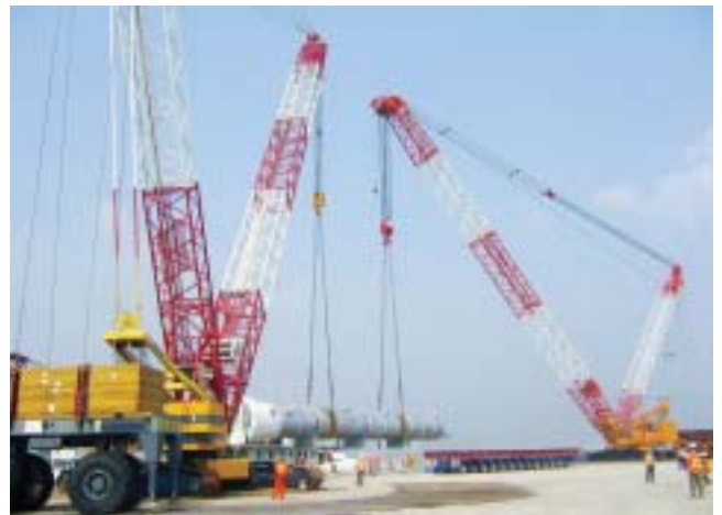
Our 550-ton and 300-ton heavy cranes performing a tandem lift at the Marine Offloading Facility in Nanhai, China.
