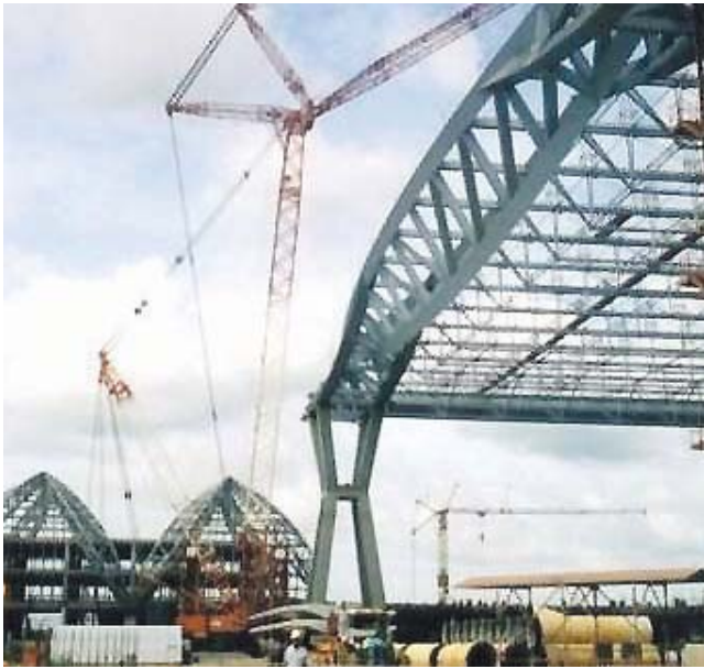
500-ton heavy crane working at The Second Bangkok International Airport in Thailand.
